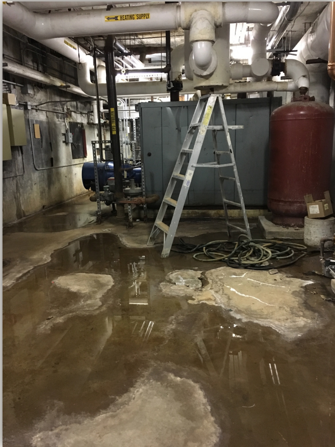
Smith Boiler Room
