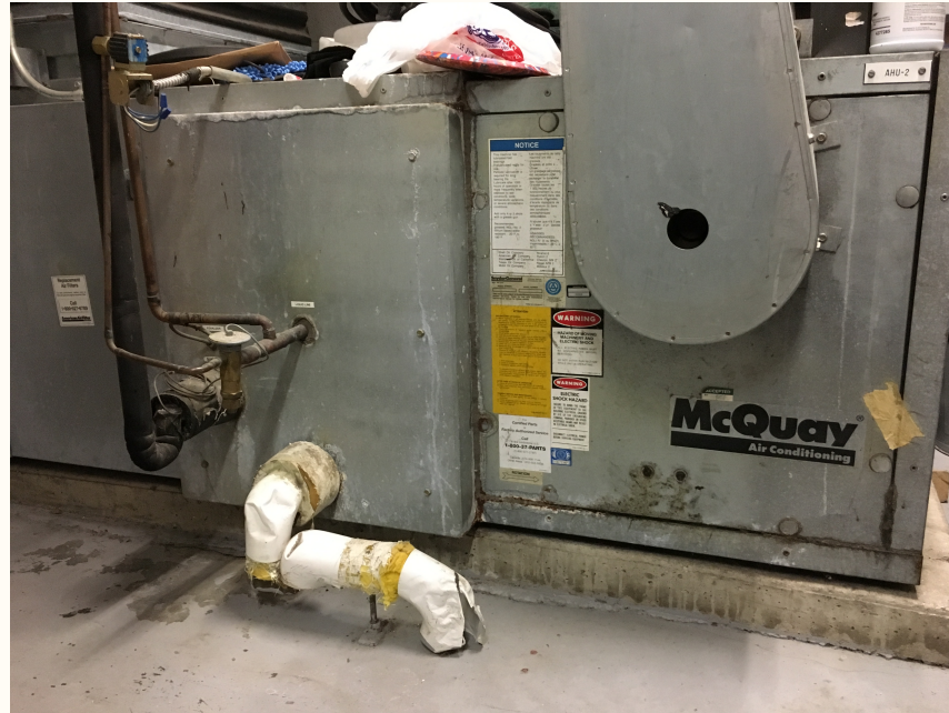
Air Conditioning Unit
